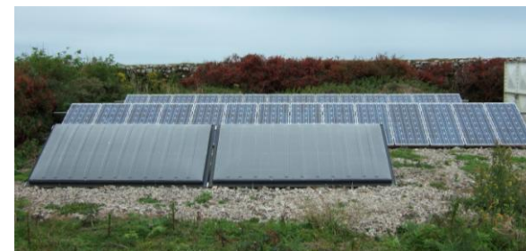
Some of the panels providing hot water and electricity situated behind the buildings
